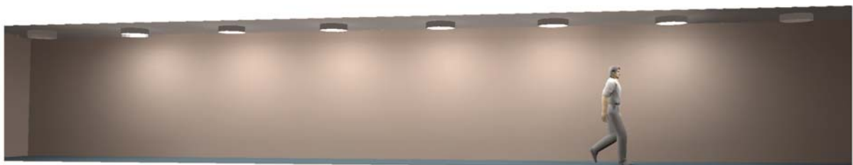
As you move along the corridor and the activation time elapses on the first fittings they dim back down to their pre-set dimming % (eg 10%).
